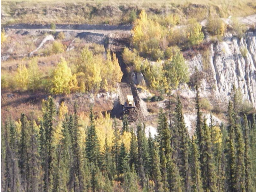
Photo 3. View of bulldozer pushing fill material down the slope. Note that berm location is in the valley behind the trees (in the foreground).
