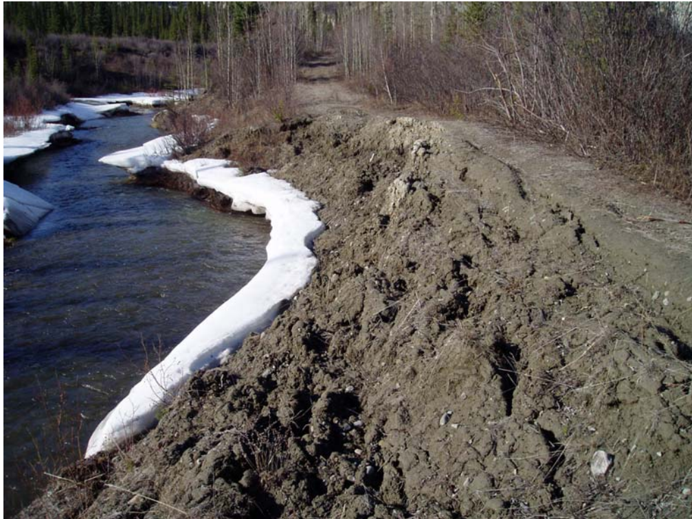
Photo 2. Downstream view of McIntyre Creek near the upstream end of berm. Significant erosion of the berm has occurred at this site.
