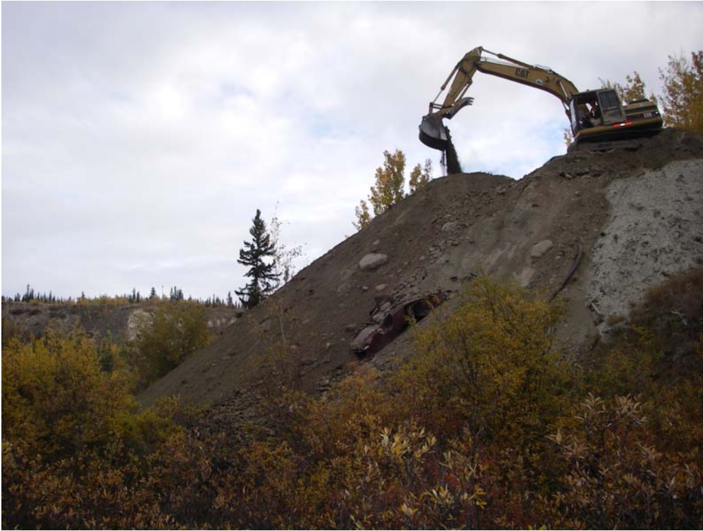
Photo 5. Excavator bailing material over slope. Proposed berm location to the bottom left of the photo.
