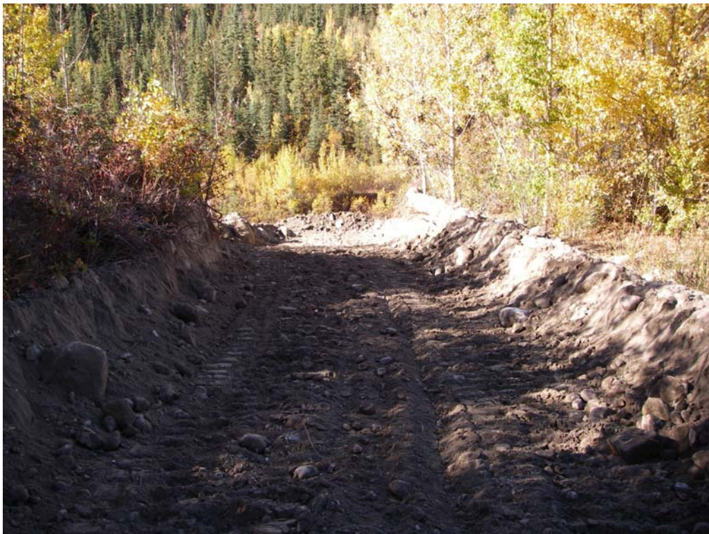
Photo 4. Downslope view of path used by bulldozer to push material down slope.
