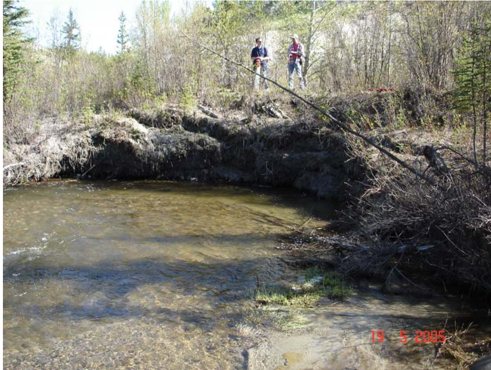
Photo 1. Downstream view of McIntyre Creek at the upstream end of existing berm. Significant undercutting of the bank adjacent to the berm has occurred at this site.
